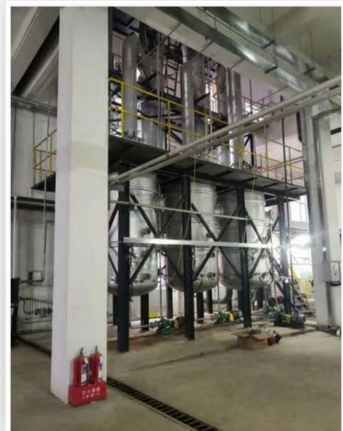
Triple-effect FM Evaporator ( Sodium Sulphate )
