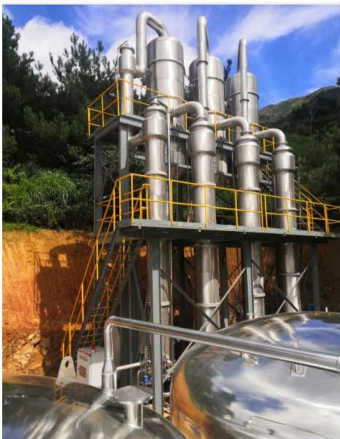
Triple-effect FC Evaporator (Distiller effluent Treatment)
