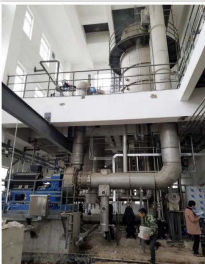
MVR Evaporator ( Landfill Leachate Treatment )
