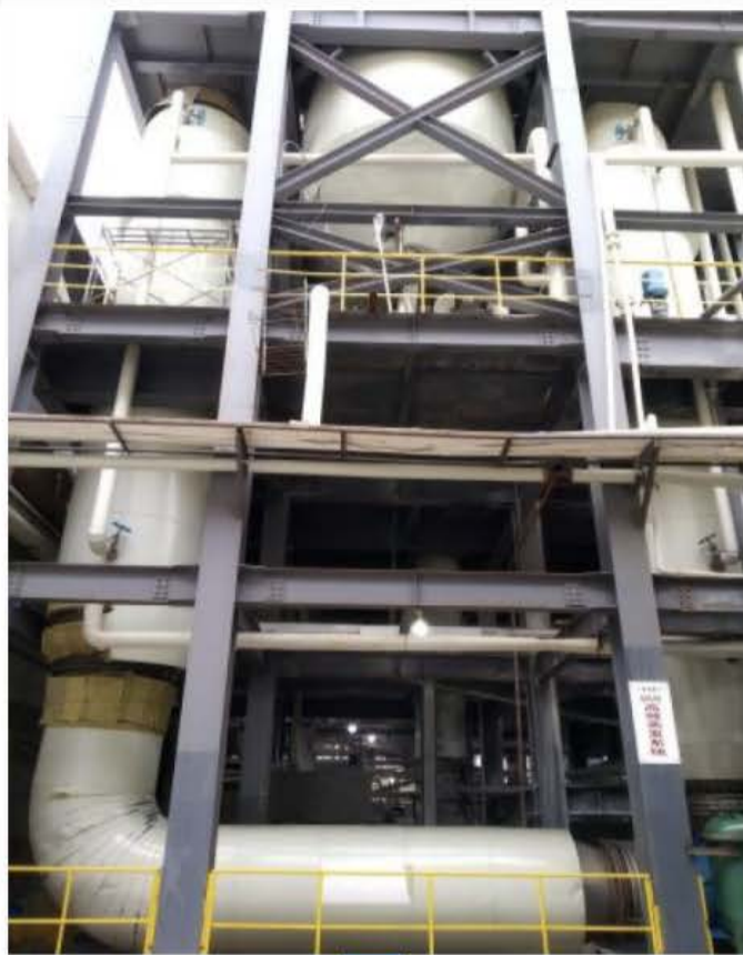
MVR Evaporator ( Sodium sulfate )
