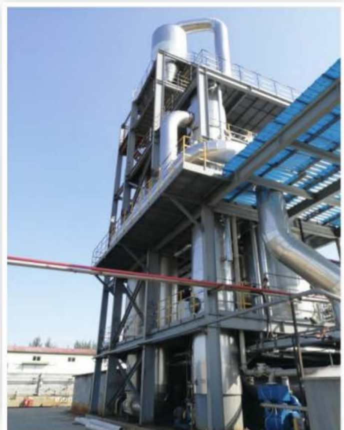
MVR Evaporator ( Ammonium sulfate )
