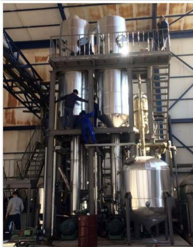
Double-effect Evaporator ( Calcium chloride )
